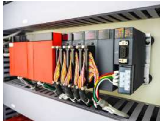
When generator gas valve is on
