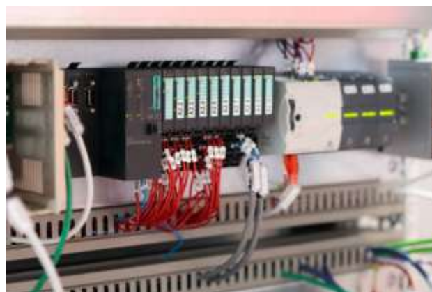
When generator at running condition
