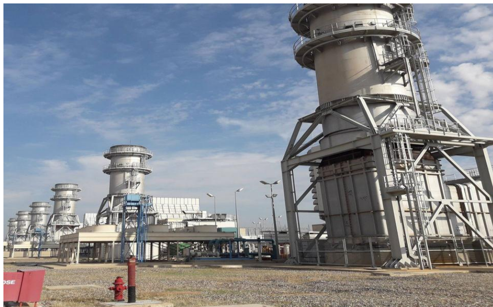
Figure 3. Qayyarah gas power station [14]
